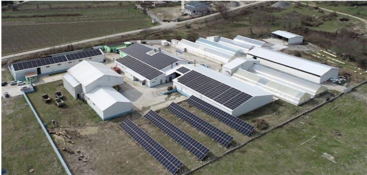
Figure 8 - PV-system at Georgian raw material partner
