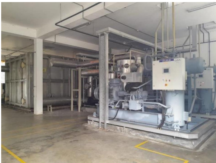
Figure 14 - Chiller system, MartinBauer, Sri Lanka
